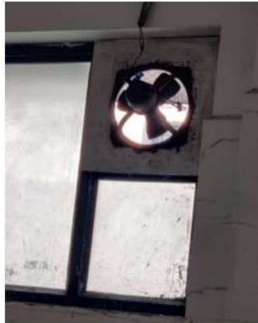
FIGURE 58: EXHAUST FAN IN TOILETS
