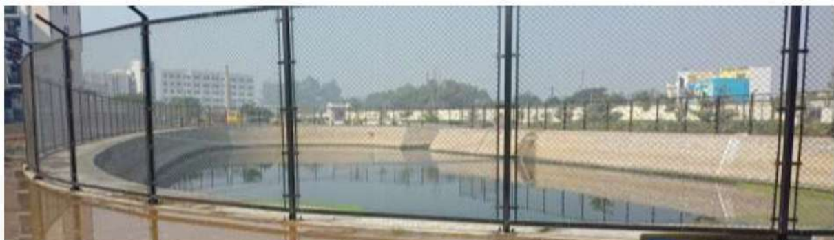
FIGURE 20: STP TREATED WATER & RAIN WATER STORAGE TANK ( CAPACITY: 1 CR. LIT)
