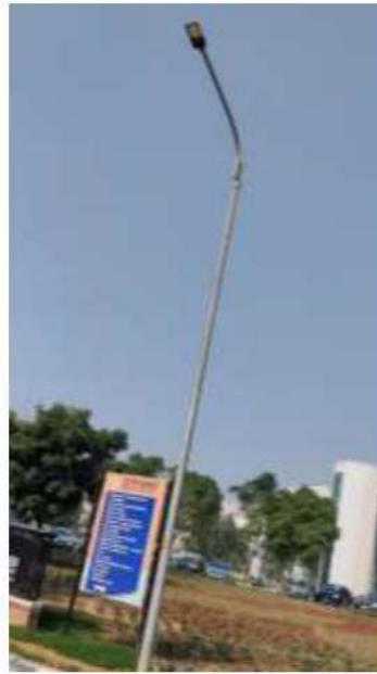
FIGURE 47: LED STREET LIGHT
