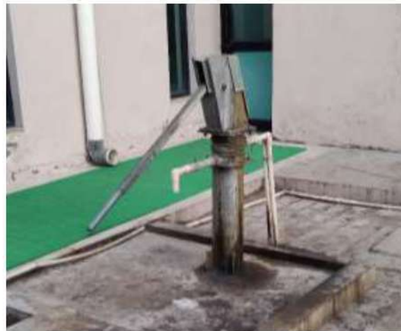
FIGURE 13: GROUND WATER EXTRACTION HAND PUMP
