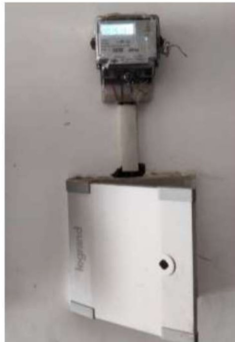
FIGURE 48: ENERGY METER AT ROOM LEVEL
