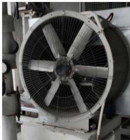
FIGURE 80: FRESH AIR FAN
