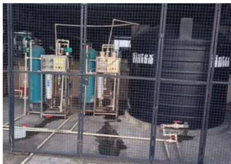
FIGURE 14: RO SYSTEM AT BUILDING TERRACE
