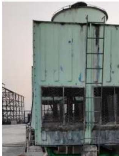
FIGURE 81: COOLING TOWER-HOSPITAL BLOCK
