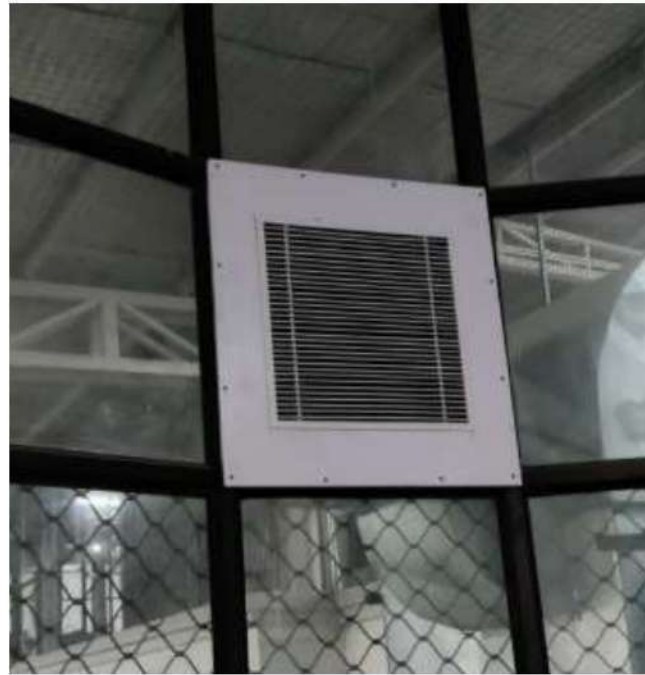
FIGURE 79: FRESH AIR GRILL -STAIRCASE
