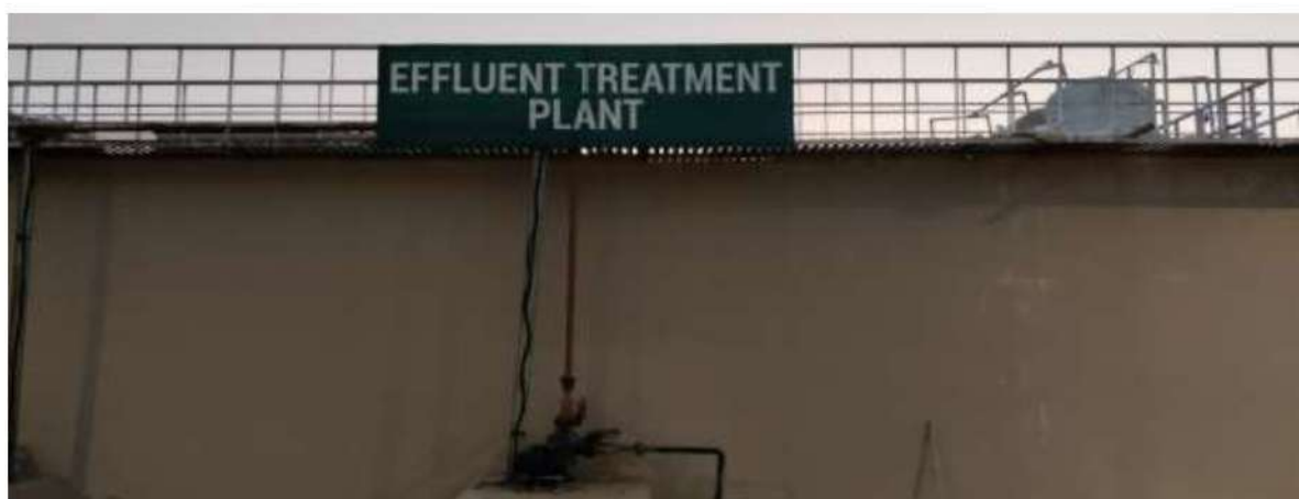
FIGURE 21: ETP FOR TREATING HOSPITAL LIQUID WASTE
